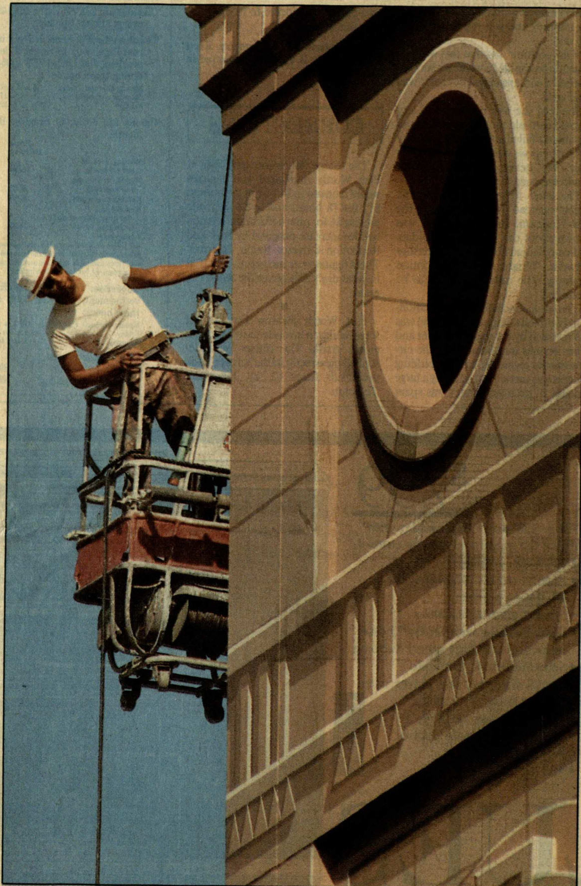
W alter Ditman, who works for American Illusion of New York, checks out the painting done on the Tarrant County Civil Courts Building
