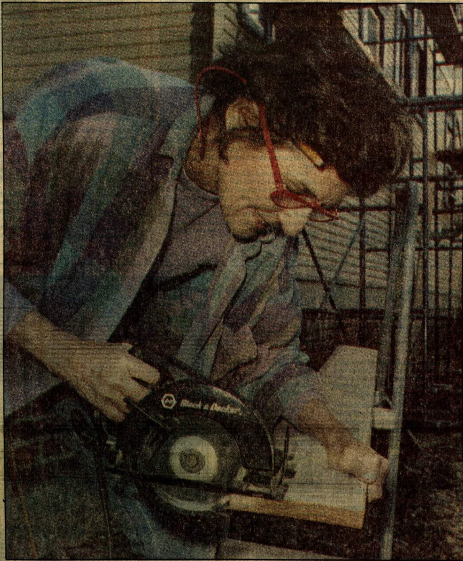
Mary Odom saws a board to frame a bathroom door at the Briggs' home, which she is restoring.
