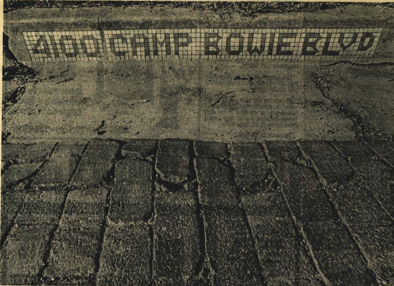
There's a shortage of brick to replace the old, worn and broken bricks on Camp Bowie Boulevard.
