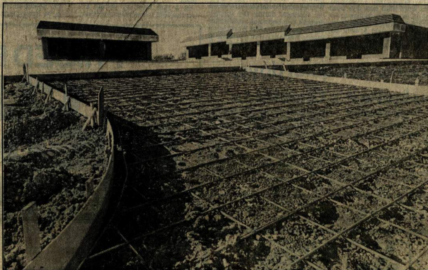
METAL REBAR... waits for cement to be poured over it at a site on Highway 114.
