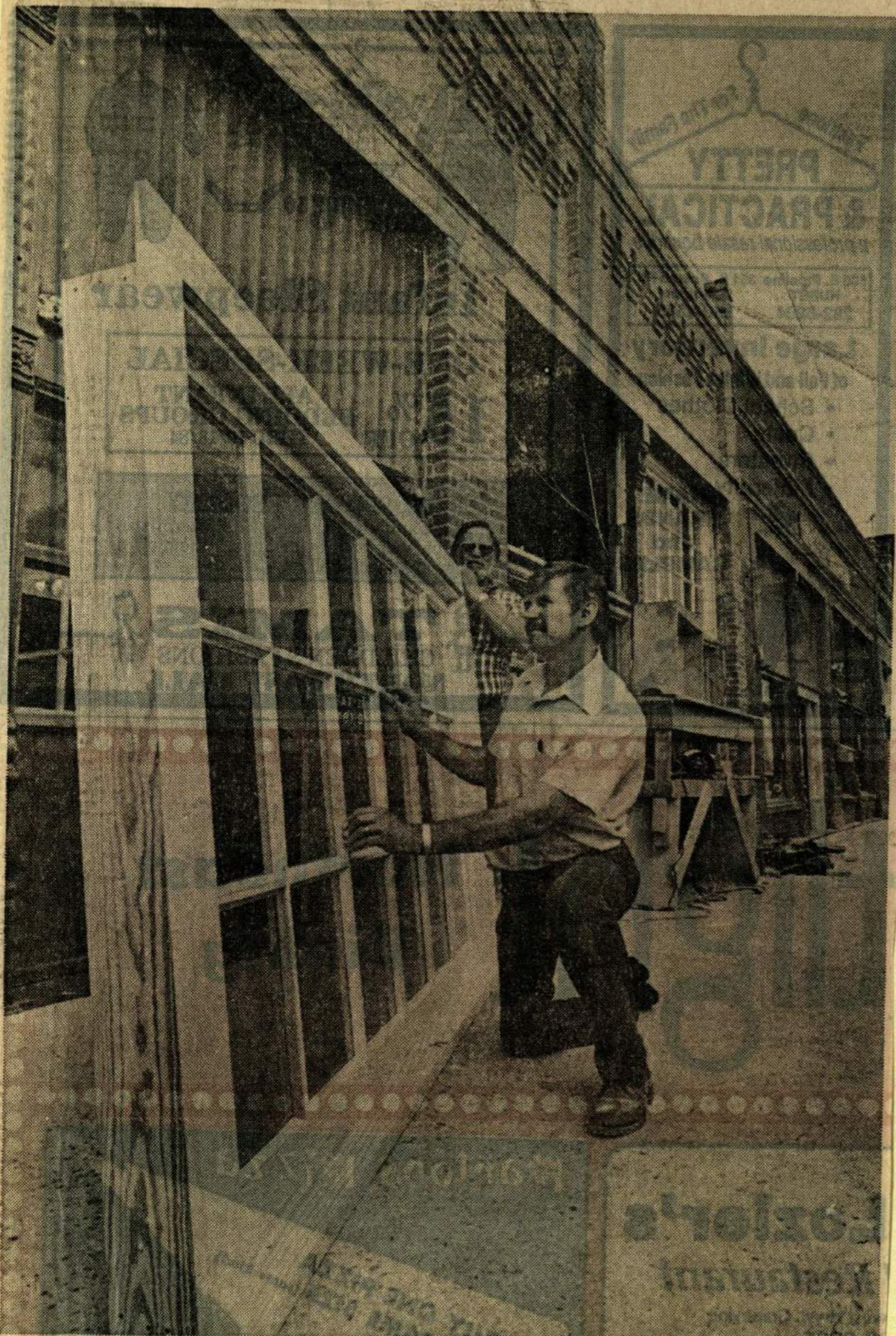
JACK CHASTEEN, LEFT, helps Doug Chasteen install new window in Off-Main Gallery in Grapevine for the renovation of the city's downtown and business district. Star-Telegram/WILLIS KNIGHT
