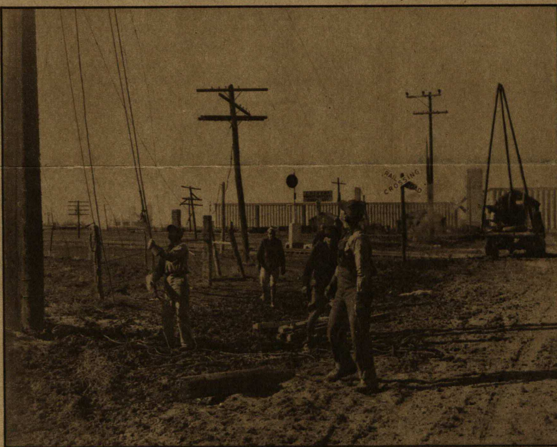
EMERGENCY CREWS went to work untangling the mass of power and telephone lines and replacing broken poles.
